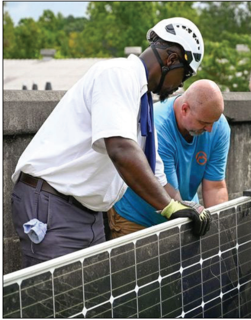
Tavaris Veal of Baldwin County, left, and Jonathan Lenz of Jones County inspect a solar panel at Baldwin County's Water Treatment Plant.
