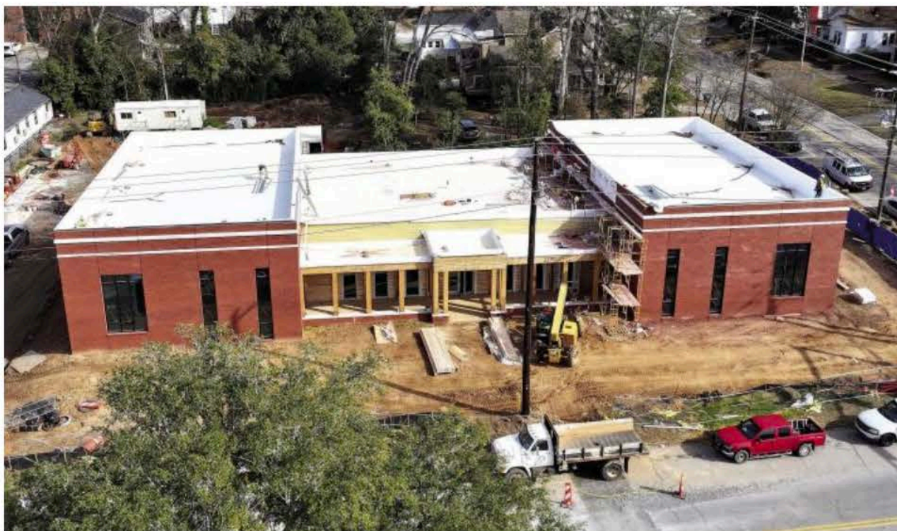
Construction of the music rehearsal hall began in July of 2024, official planning began two years prior. The goal is to have the facility open to students by next fall semester. Scan the QR code to see a video of the building by Georgia College. COURTESY OF GCSU
